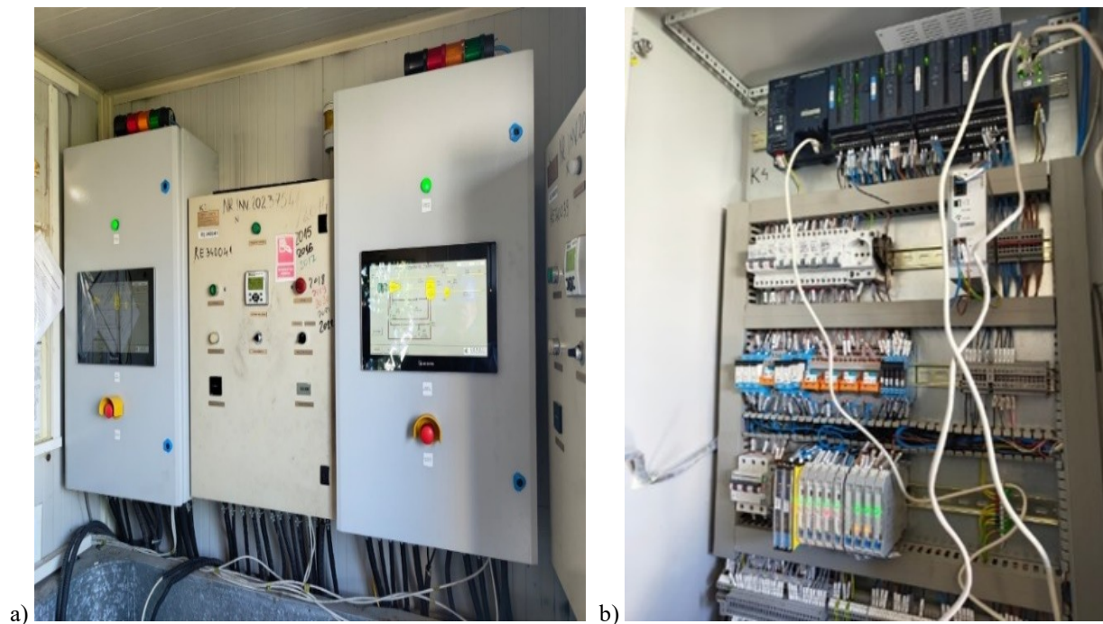
Fig. 2. a) The four automation cabinets, first and third from left to right b) The interior of one of the modernized automation cabinets
