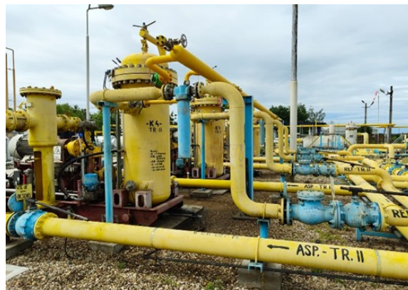
Fig. 1. Stoenеști gas compression station
