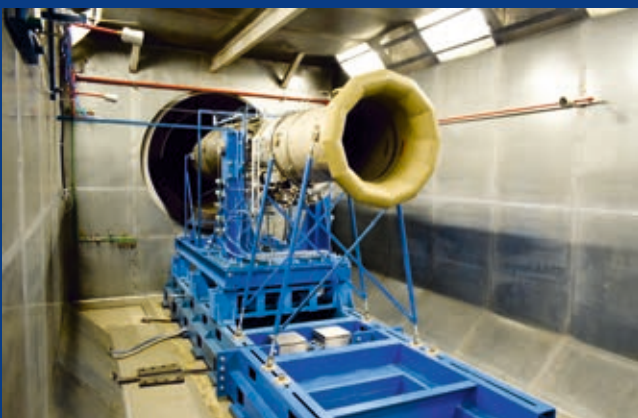
Test Cell no.2-Turbojet or turbofans engines testing facilities
