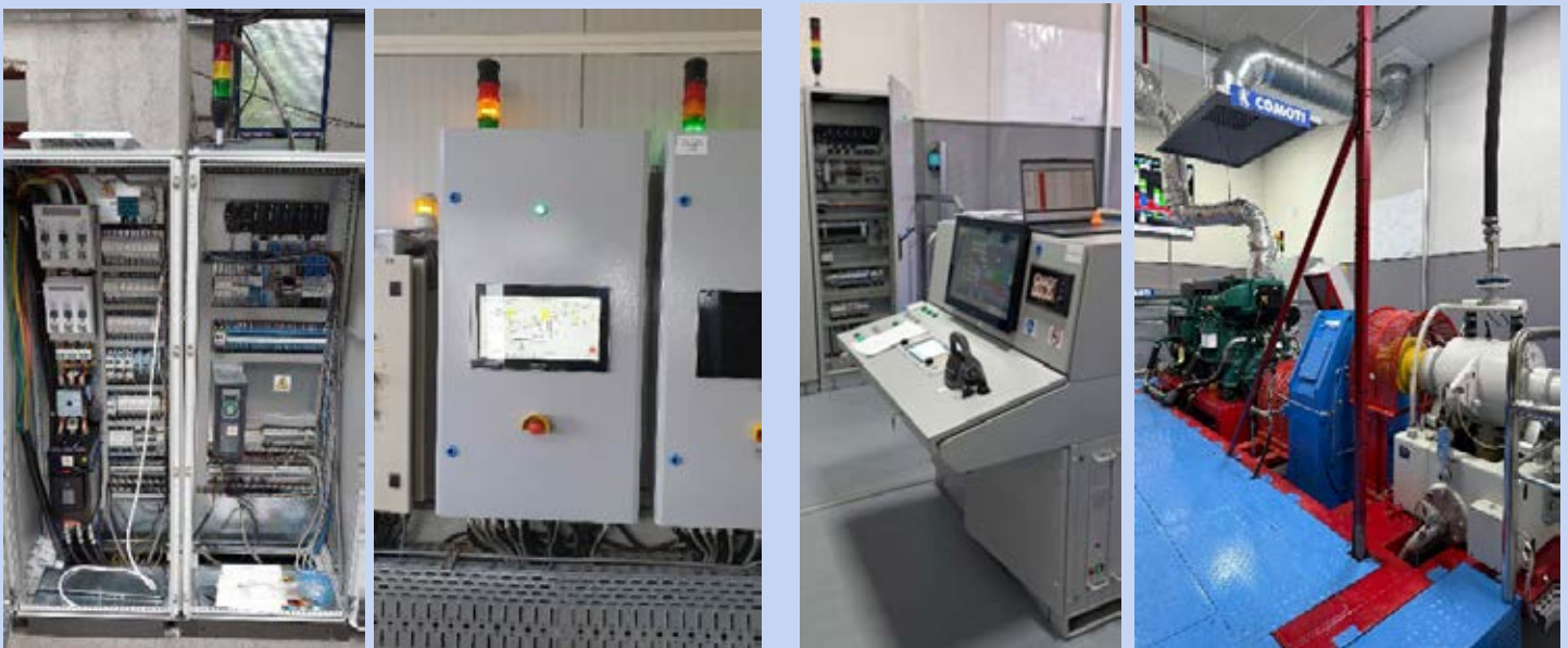
Automation cabinets for compressors, installed in control rooms within stations for oil and gas industry
