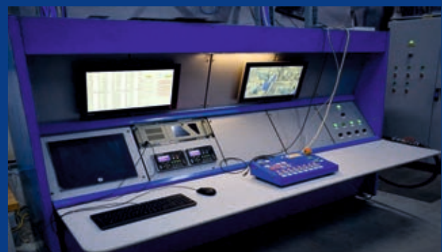
Auxiliary control and instrumentation unit.
