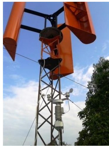
Figure 15. Lenz wind turbine – closer look.
